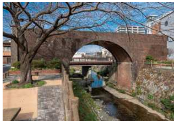
5 Kyushu Railroad bridge in Chayamachi Address: 4, Chayamachi, Yahatahigashi-ku Built in 1891 Blueprint: unknown
